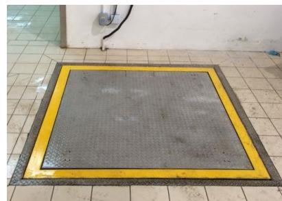
LF-DS stainless steel floor scale installed in pit
